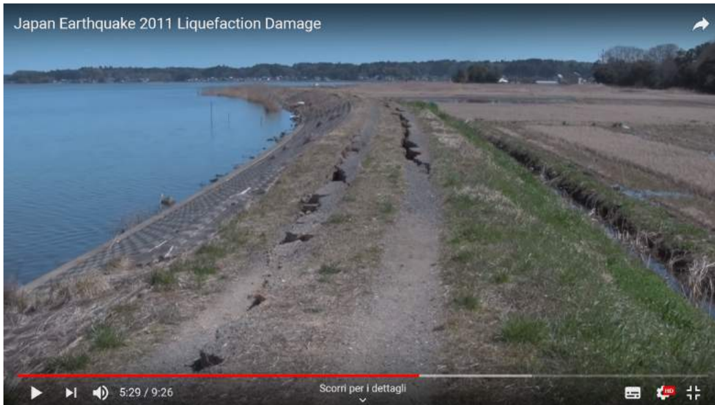
Figure 1-9: Cracking of levees (OSU, 2011).
