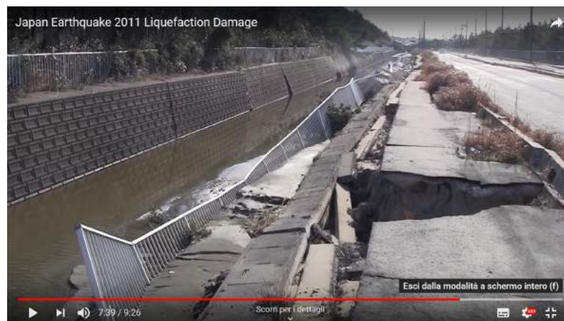
Figure 1-6: Collapse of earth retaining structures (OSU, 2011).
