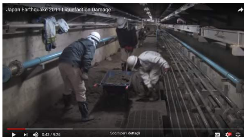
Figure 1-2: Extensive sand ejecta in open areas and at the basement of a treatment plant (OSU, 2011).
