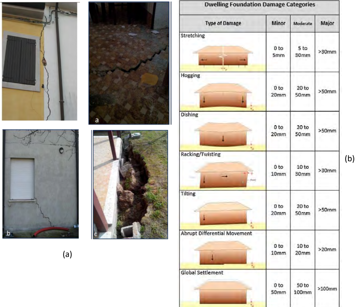
Figure 5-21 Examples of the most typical liquefaction-induced building damage in the municipality of Terre del Reno (a) and criterium adopted for the classification of damage (b) from van Ballegooy et al., 2014.
