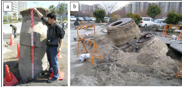
Figure 6-2 Uplift of sewage manholes caused by liquefaction.
