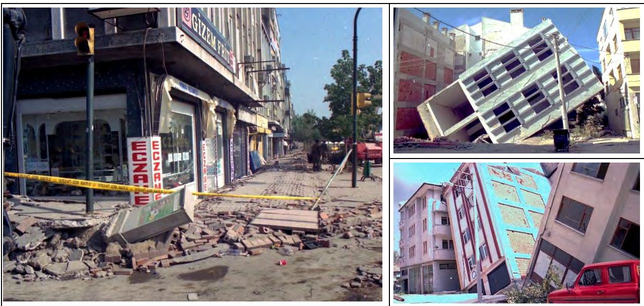
Figure 4-1: Typical photographs-1 for buildings with Liquefaction Induced Damage (LID) (Provided by Adapazari and Sakarya Municipalities and taken during site visits).
