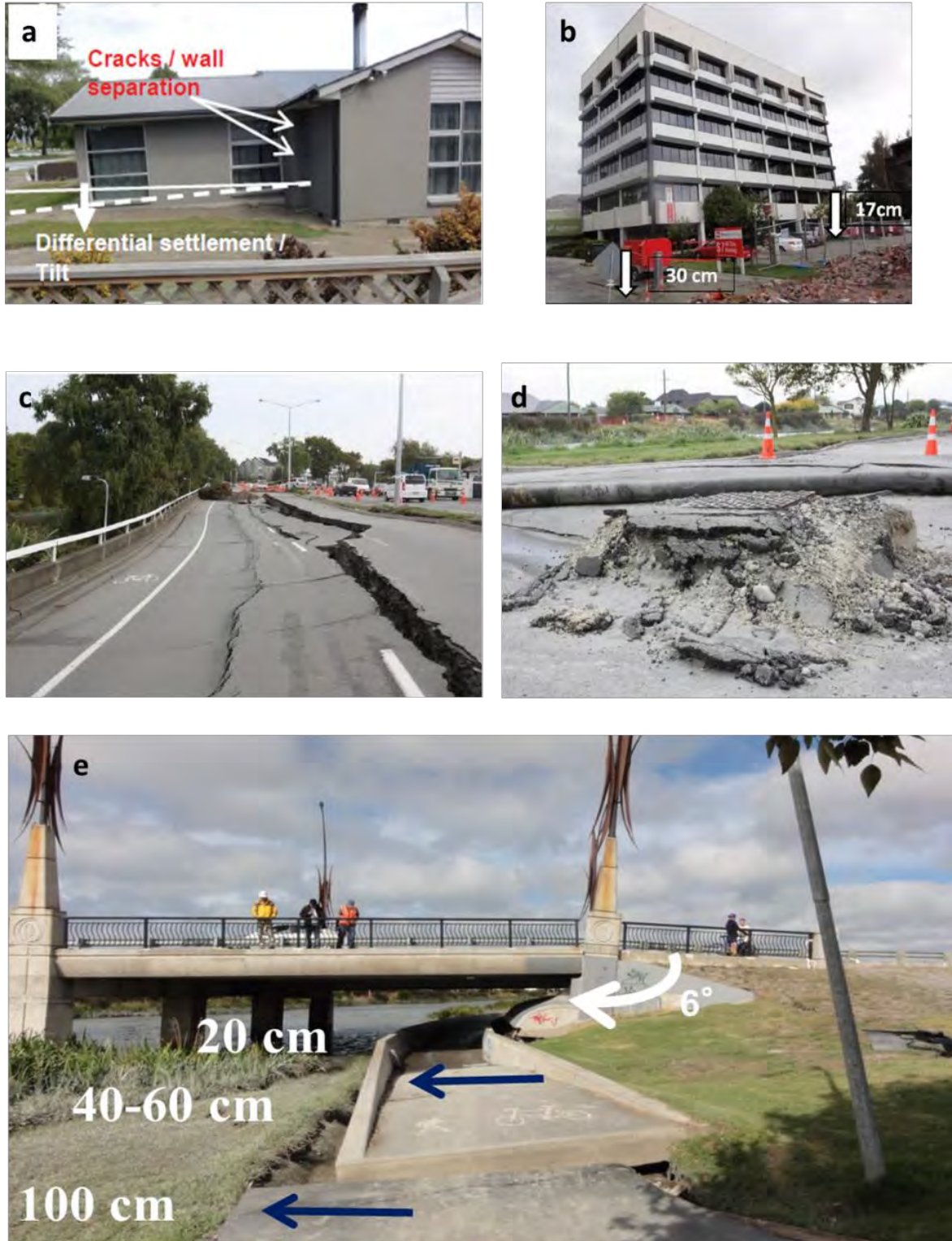
Figure 3-2 a) differential settlement resulting in tilt and damage to residential house (Cubrinovski et al., 2012); b) Building on pile foundations in area of severe liquefaction showing large settlement of the surrounding soils relative to the foundation beams (Cubrinovski et al., 2011a); c) Effect of lateral spreading on the roadway (Goldsworthy, 2012); d) Flotation of pipe below causes the manhole to rise (Goldsworthy, 2012); e) Rotation of bridge abutments.
