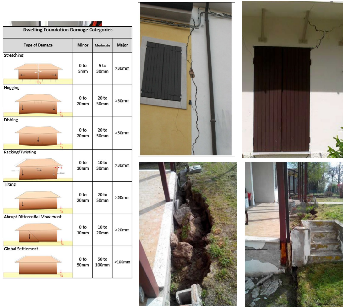
Figure 7.2: Indicative building damage caused by an EILD event
