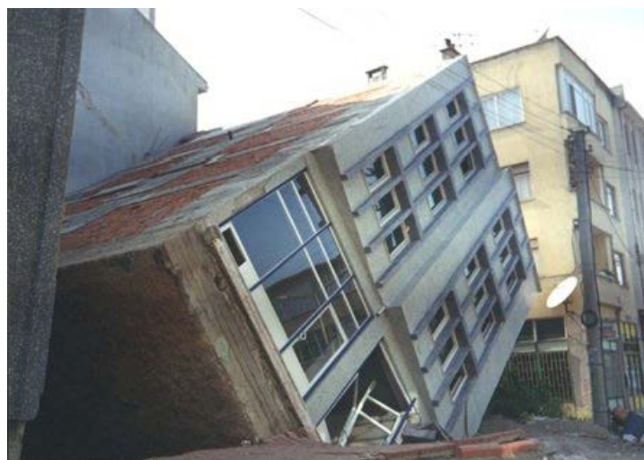
Figure 2-11 Overturned building due to liquefied foundation, Izmit, Turkey 1999 (Erdik et al., 1999)
