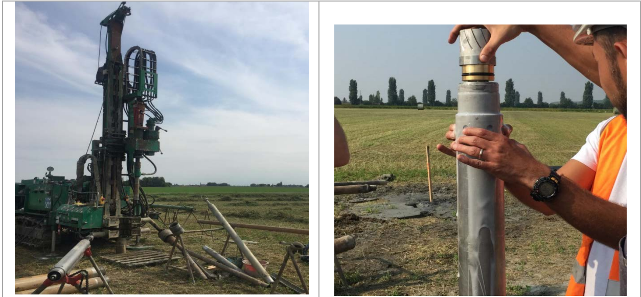
Figure T4.3.1. . Photos of the in situ investigation in Pieve di Cento (BO, Italy)
