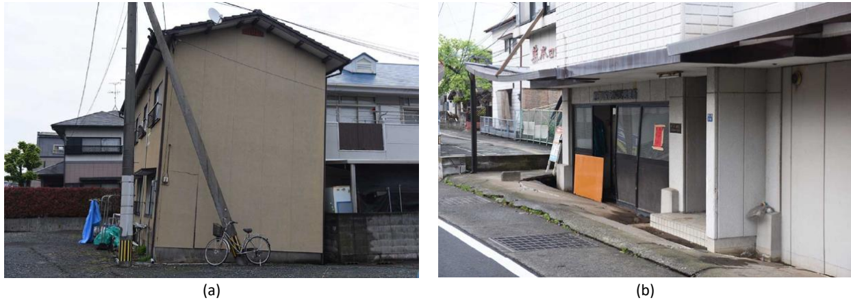
Figure 1.6: (a) Liquefaction-induced tilt of a 2-storey wooden house in Karikusa town; (b) Liquefaction-induced settlement of a 3-storey reinforced concrete building in Karikusa town (Tokimatsu et al., 2017)
